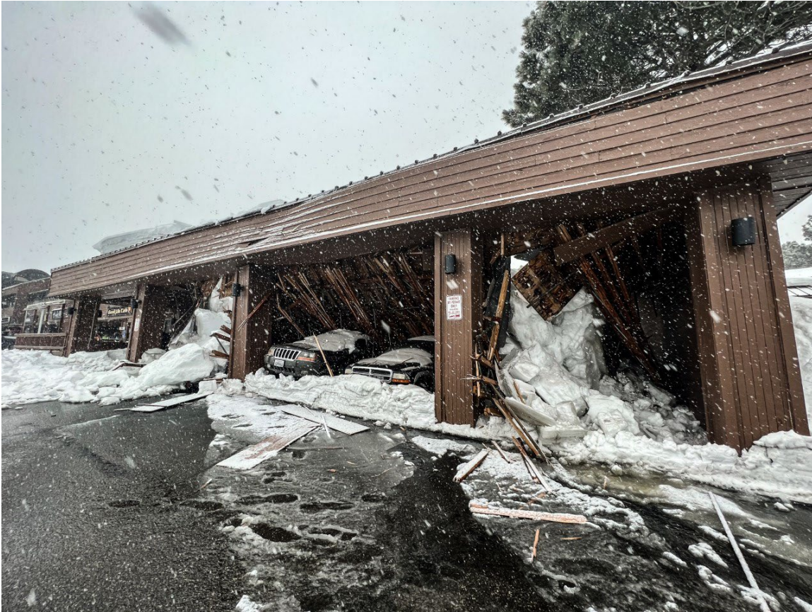
Figure 2: Collapsed Structure during a Winter Storm, 2023
