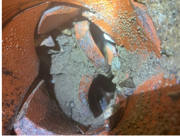
Figure 2: Broken Water Main Pipe at a Depth of 21 ft in a Congested Area of June Lake 1
